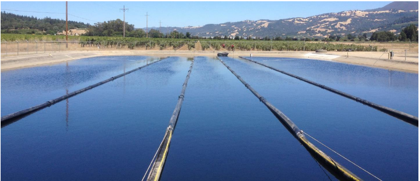
Fine Bubble Diffuser Aerated Wastewater Treatment Technology Installed in Pond
